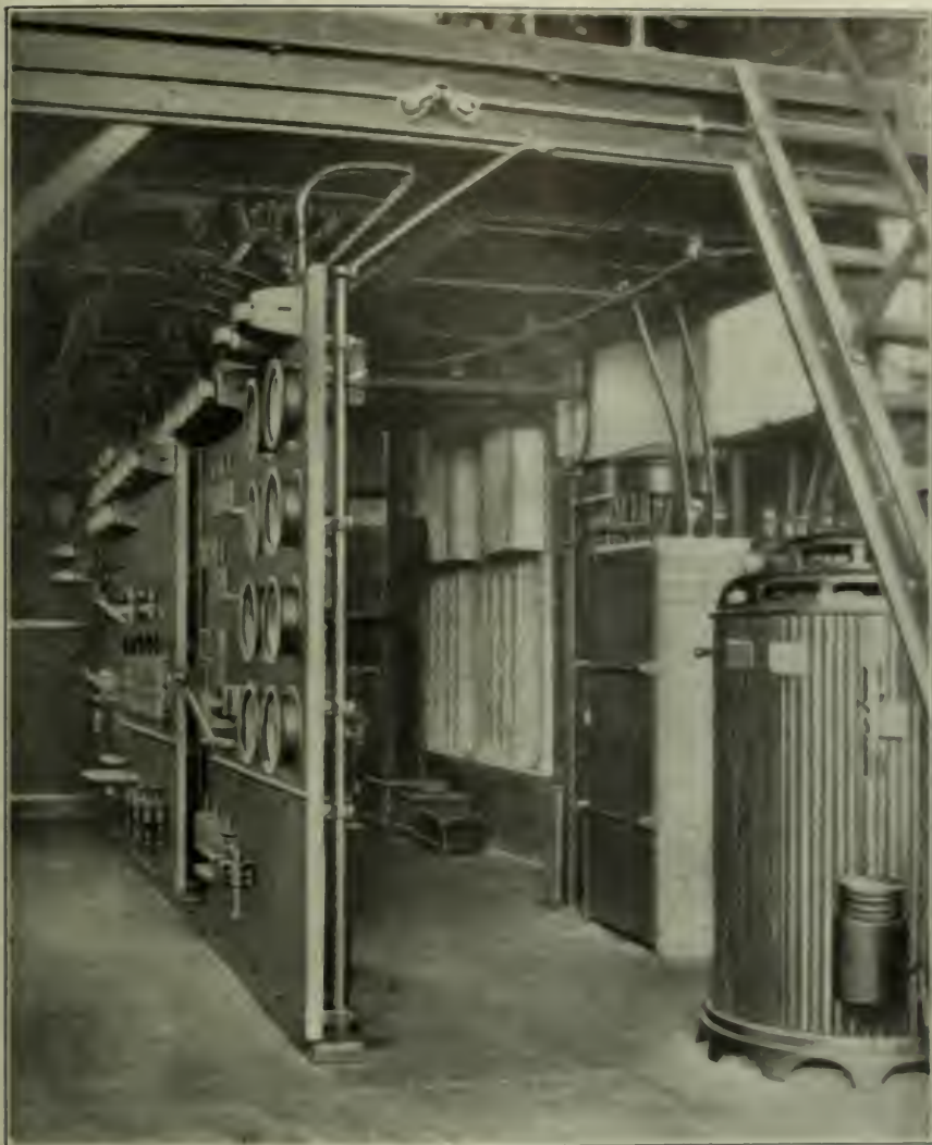
FIG. 5 SWITCHBOARD IN POWER STATION
